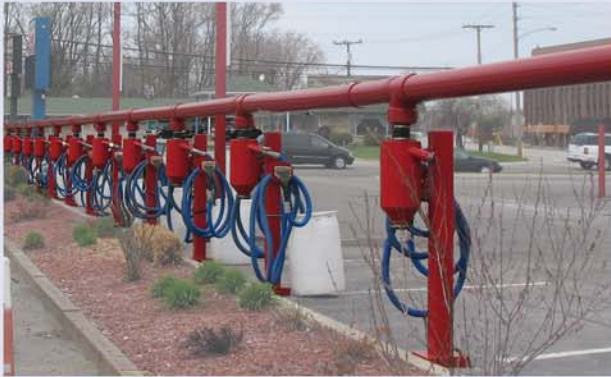
Hopper Stanchions with overhead piping, Easy Clean Car Wash, Lansing, Chicago
