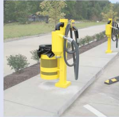
Hopper Stanchions with buried pipe, Suds Soft Touch, Corbin, KY
